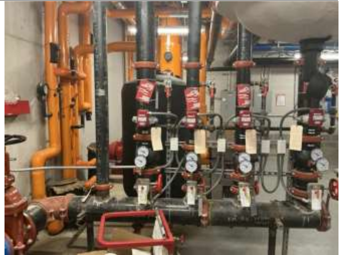
26 - FIRE SUPPRESSION SYSTEM
