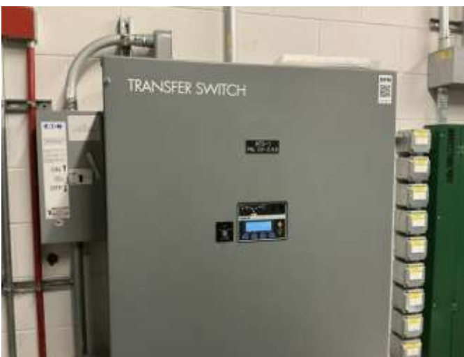
29 - AUTOMATIC TRANSFER SWITCH
