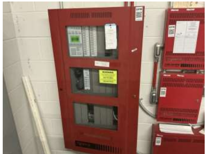
28 - FIRE ALARM PANEL
